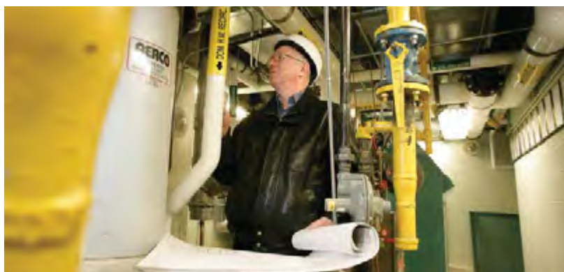
Geothermal heating and cooling at the Richmond Hill Centre for the Performing Arts
