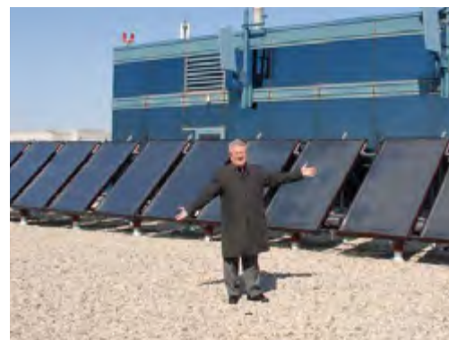
Solar water heating system at the Richmond Hill Municipal Offices
