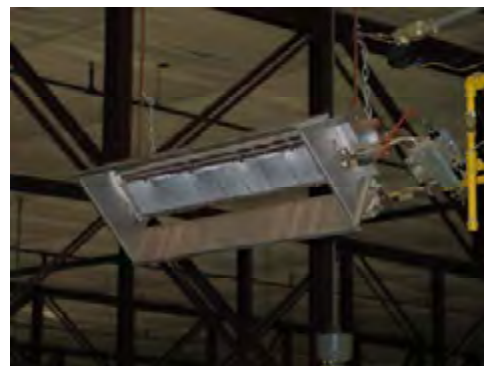
Note in this picture that the radiant panels are surrounded by an open air path which creates convection cooling of the panels reducing the amount of radiant energy generated. Air warmed by the panels moves toward the ceiling – not warming the spectators. There are new high intensity IR panels that minimize this convection cooling effect and offer higher overall efficiency. Upgrade to new heaters could be considered depending upon level of use. Note that mounting height evaluation is crucial with higher efficiency units.
