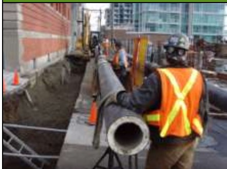
Adding to the LEC pipeline network. Photo courtesy of the City of North Vancouver.
