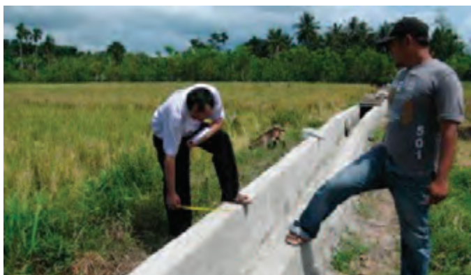
An infrastructure specialist from CALGAP provides technical assistance to the Cinta Damai farmers group on an irrigation project.
